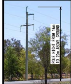
VIEW OF 66kV POLE
