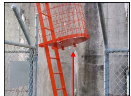
Ladder Security Guard Locked Closed
