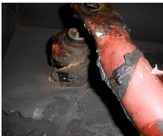
Fig 6 – Close up of the damage to the end of the Bushing and the cable termination. (The rear plate of the endbox is still in position)
