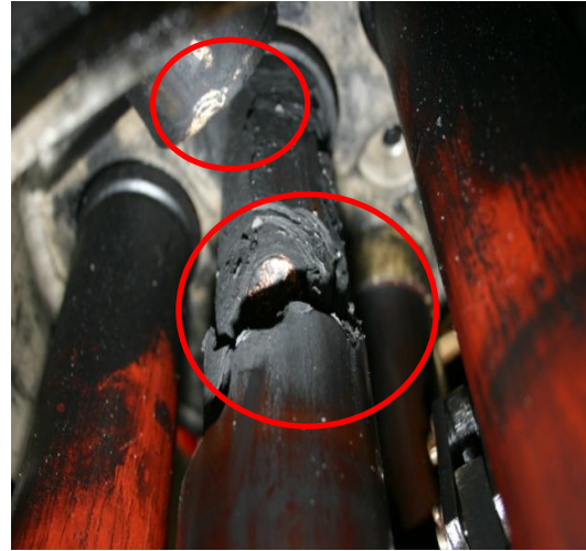
Fig 2 – Evidence of Flashover from Bushing to Tank
