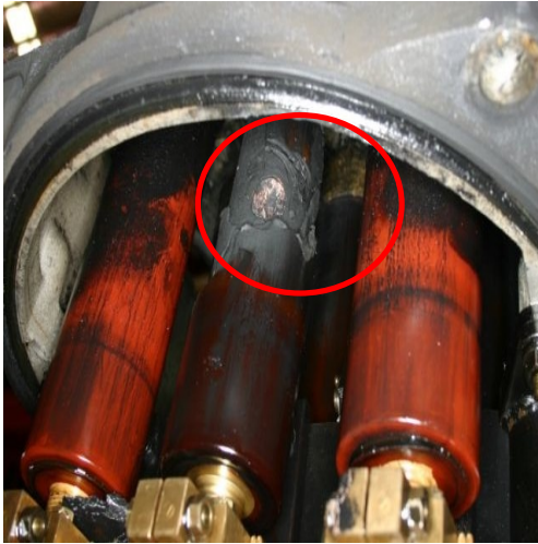
Fig 1 – Damage to Circuit Breaker Bushing
