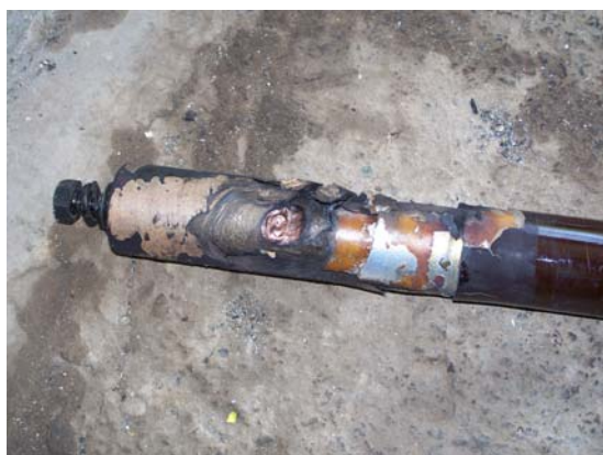
Fig 2 – Close up of the damaged bushing showing the position of the puncture through the bushing insulation.
