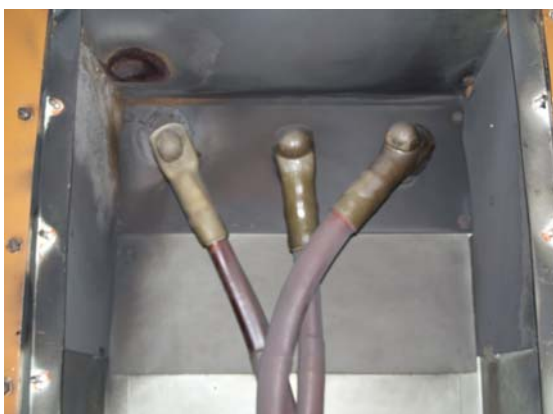
Fig 1 – View of the endbox showing the cables bolted to the ends of the bushings and covered by heat shrink boots. The failed bushing is in the left. Note the burn mark above.
