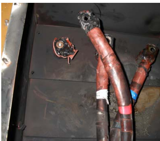
Fig 5 – View of the endbox. The damaged C phase bushing is on the (LHS). The cables have been unbolted from the bushings. The heat shrink boots have been removed.
