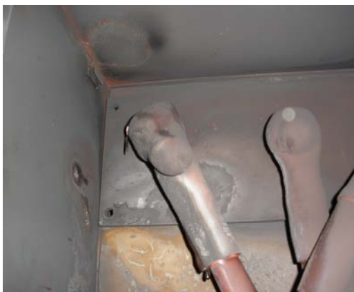
Fig 3 – View of the endbox showing the cables bolted to the ends of the bushings and covered by heat shrink boots. The damage to the LHS cable end and insulating boot is apparent.
