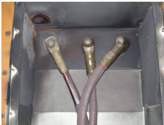
Fig 5 – View of the endbox showing the cables bolted to the ends of the bushings and covered by heat shrink boots. The failed C phase bushing is on the left. Note the burn mark above.
