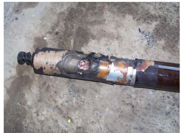
Fig 6 – Close up of the damaged bushing showing the position of the puncture through the bushing insulation.
