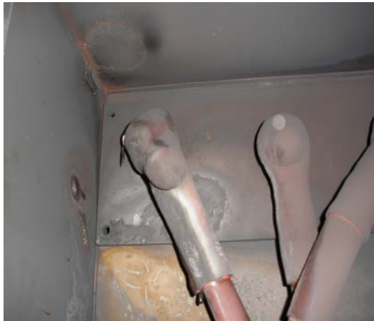
Fig 11 – View of the LHS of the endbox showing damage and missing components.
