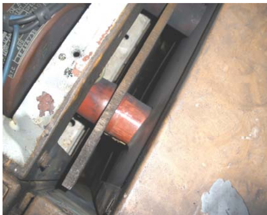
Fig 15 – View from the top, showing that the endbox has come adrift from the CT chamber by approximately 7.5 cm.
