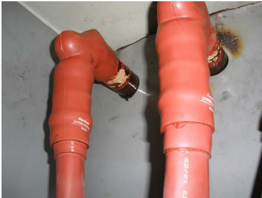
FAC Feeder Endbox bushings and cable terminations. (A and B phase only).
