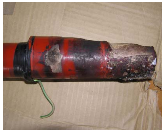
Fig 9 – View of the damaged C phase bushing, from the other side, showing the shallow second puncture clearly visible 13.3 cm from the end.
