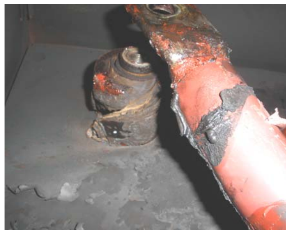
Fig 14 – Close up of the damage to the end of the C phase bushing and the cable termination. (The rear Bakelite plate of the endbox is still in position)
