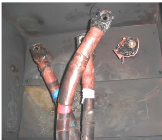
Fig 13 – View of the endbox. The damaged C phase bushing is on the (LHS). The cables have been unbolted and the heat shrink boots removed.
