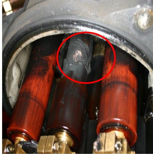
Fig 1 – Damage to Circuit Breaker Bushing at the point of failure inside the tank
