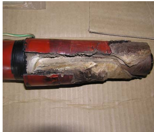
Fig 7 – View of the damaged C phase bushing, showing the full length tear.
