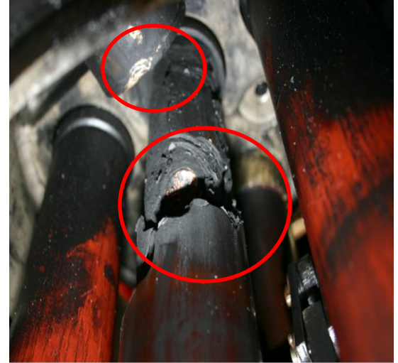
Fig 2 – Evidence of Flashover from Bushing to tank
